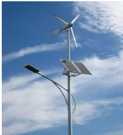
Fig. 6. Wind and solar combined system to support and power a street light
