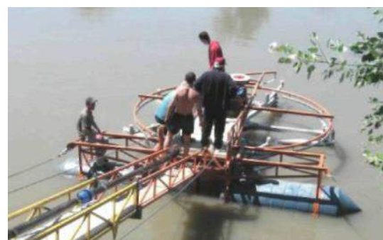
Fig. 16. The industrial prototype of the micro-hydro power plant installed on the Prut River [9]
