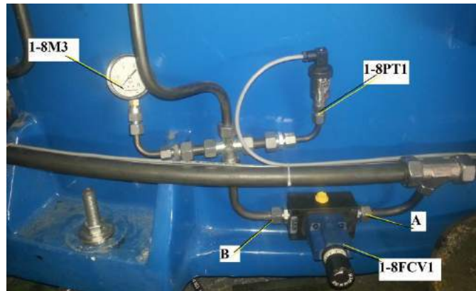
Fig. 12. Location of the control and regulation devices for the pressure in pockets
