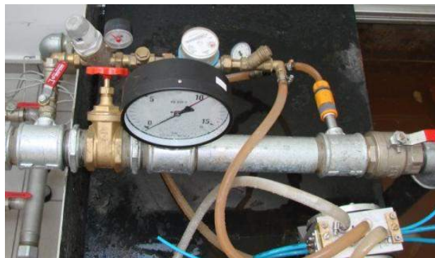
Fig. 9. Elements of control and monitoring of the working parameters
