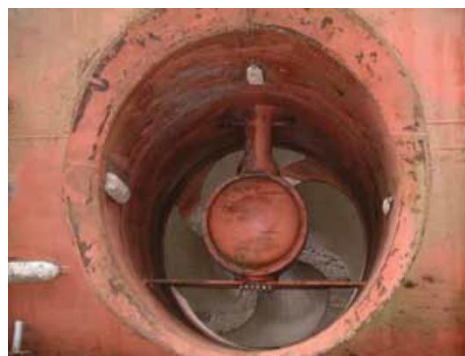
Fig. 29. Corrosion in and around thruster tunnel [30]
