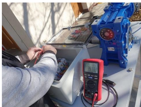
Fig. 12. Measurements of current, voltage, powers, power factor
