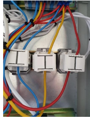
Fig. 5. Current transformers 120A
